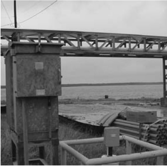
19.8 Oil immersed rectifier and deep well.
