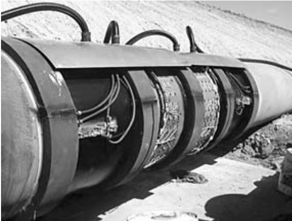
28.7 Case study 3: two FSM-IT matrices installed on adjacent new/old pipes.
