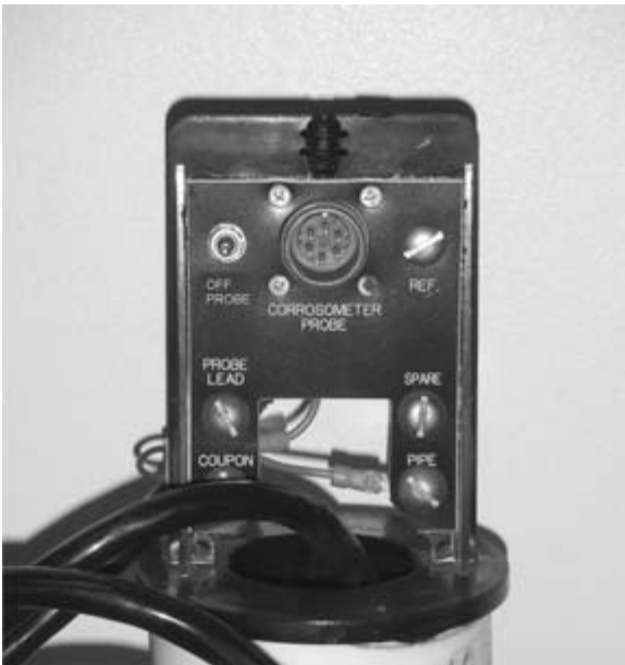
17.5 ER probe test station head.
